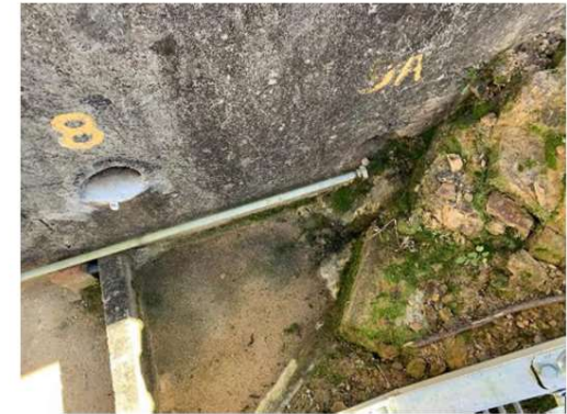
Toonumbar Dam Inject 1 – Seepage Point 8
